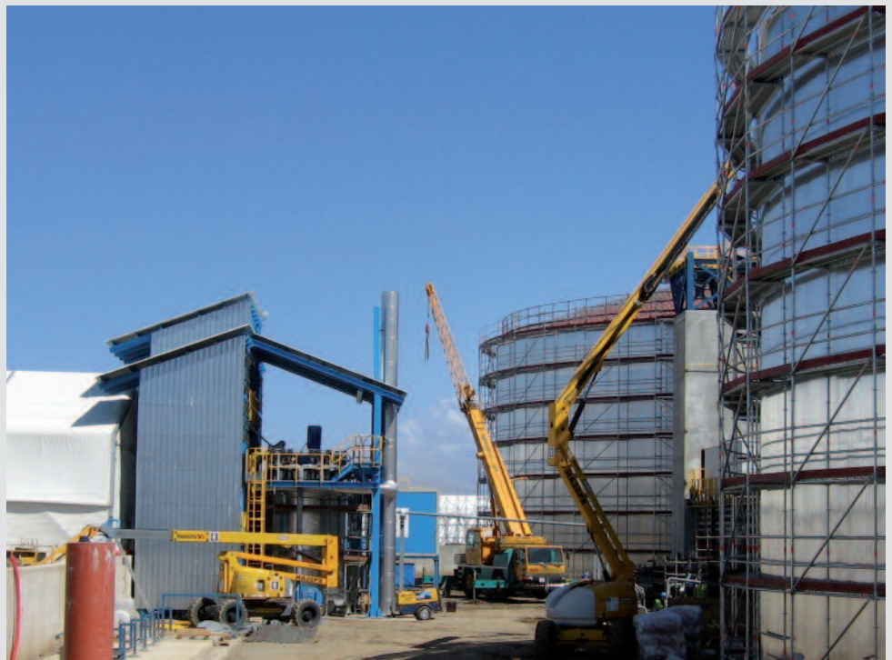
The melting furnace under construction with the two liquid salt tanks which serve as heat storage.
